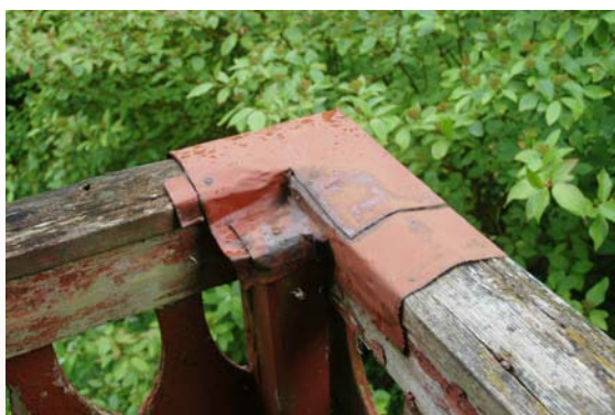
Figure 14: Fungal decay at a mitre joint
