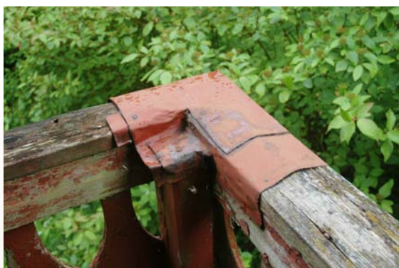
Figure 14: Fungal decay at a mitre joint
